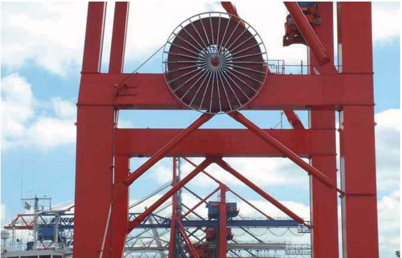
Frequency driven VAHLE Motor Reelers, container crane at Hamburg Harbour
