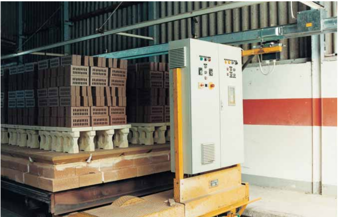
VAHLE POWERCOM®-data transmission at a brick kiln.
