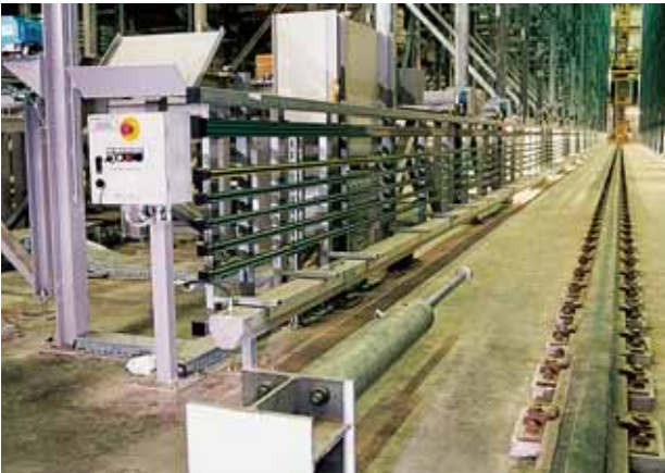
High bay warehouse with stacker crane
