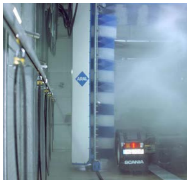
Hose-transportation in a truck washing facility
