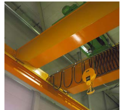
Power supply of the crab on an overhead bridge crane
