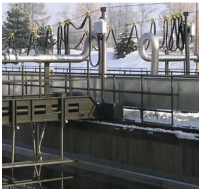
Main power supply of a longitudinal scraper bridge in a waste water treatment plant
