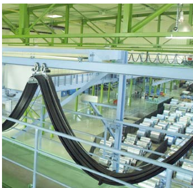
Energy and data transmission on a steel-mill-crane
