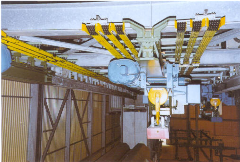
Automatic crane installation for transfer operation with pick up guides in a zinc coating plant.
