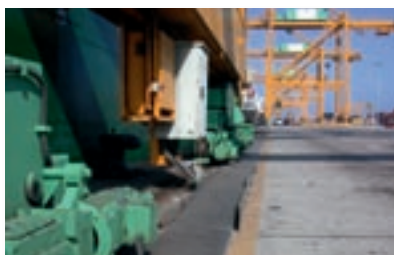
Heavy enclosed conductor system
