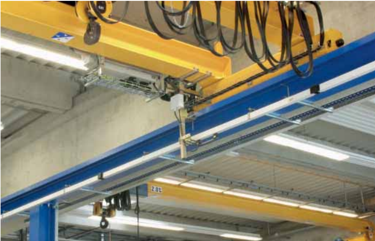
Crane installations at company Rheinmetall Landsysteme (Kiel)
